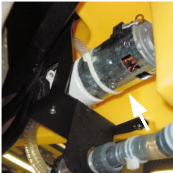
Water pump (M4)
